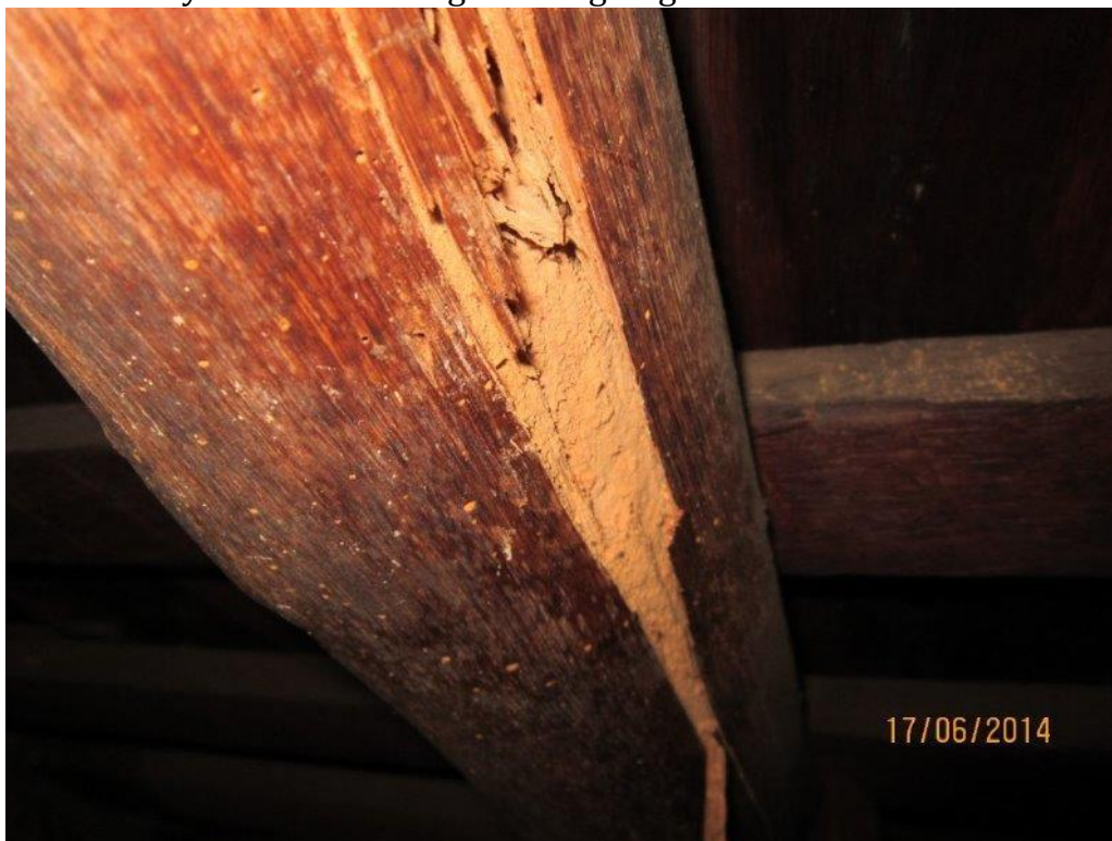
Photo 28 Lyctid borer damage turning large sections of the timber to dust.
